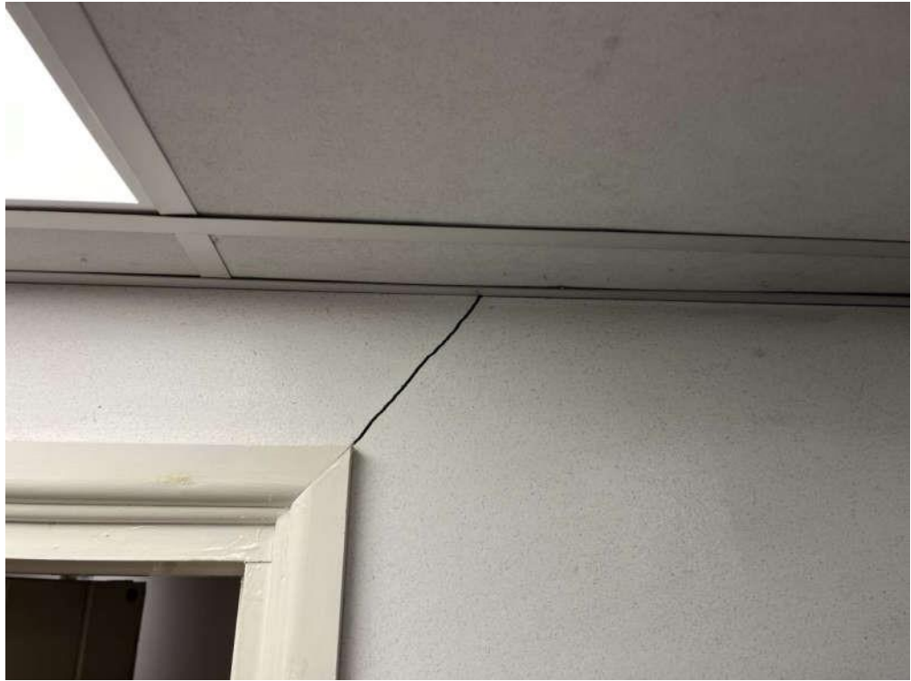
Photograph 8 – Cracking to blockwork over Ground Floor doorway.
