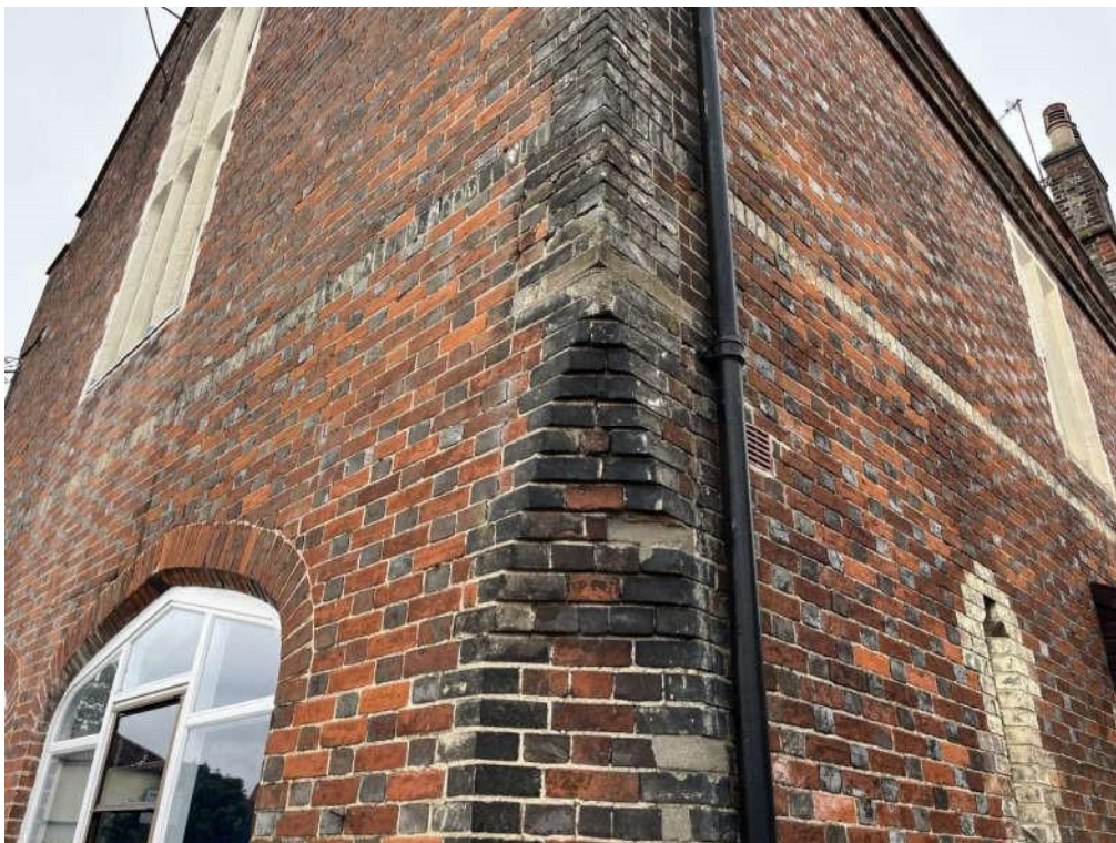
Photograph 3 – North West corner corbel (note previous cementitious repairs).
