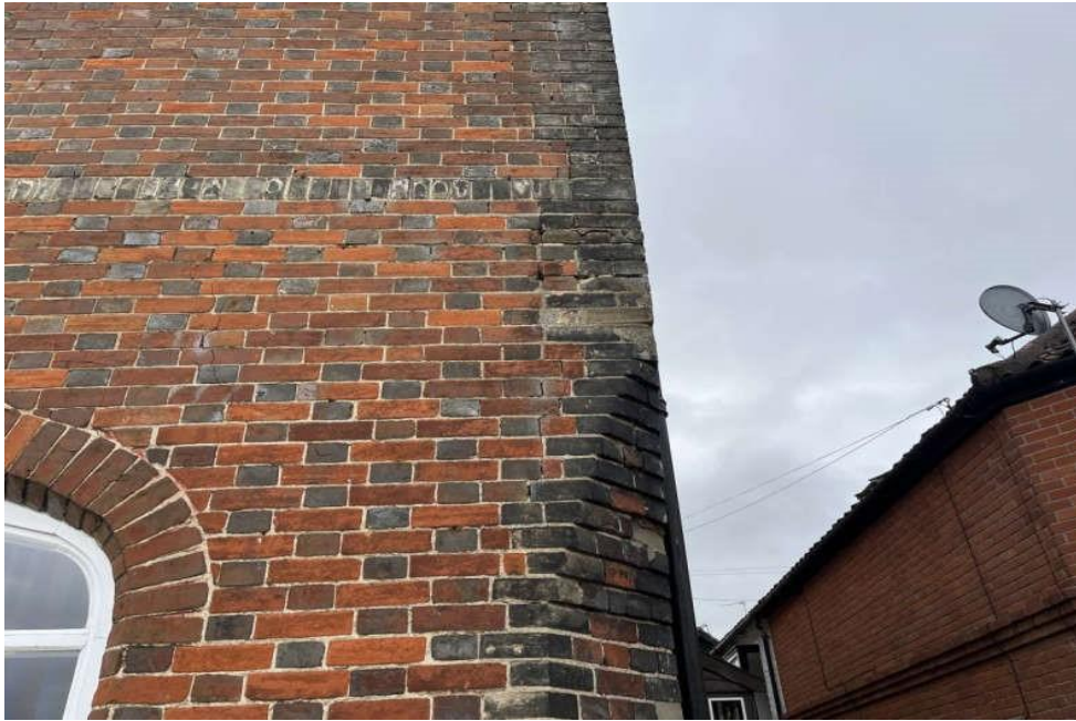
Photograph 2 – North West corner cracking.
