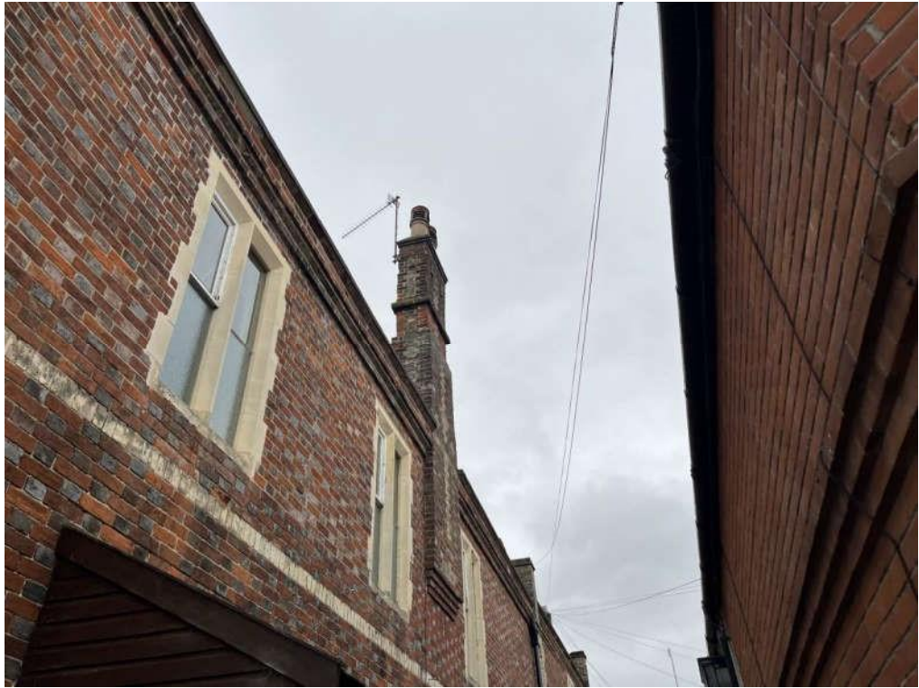
Photograph 10 – ‘Leaning’ chimney looking South.
