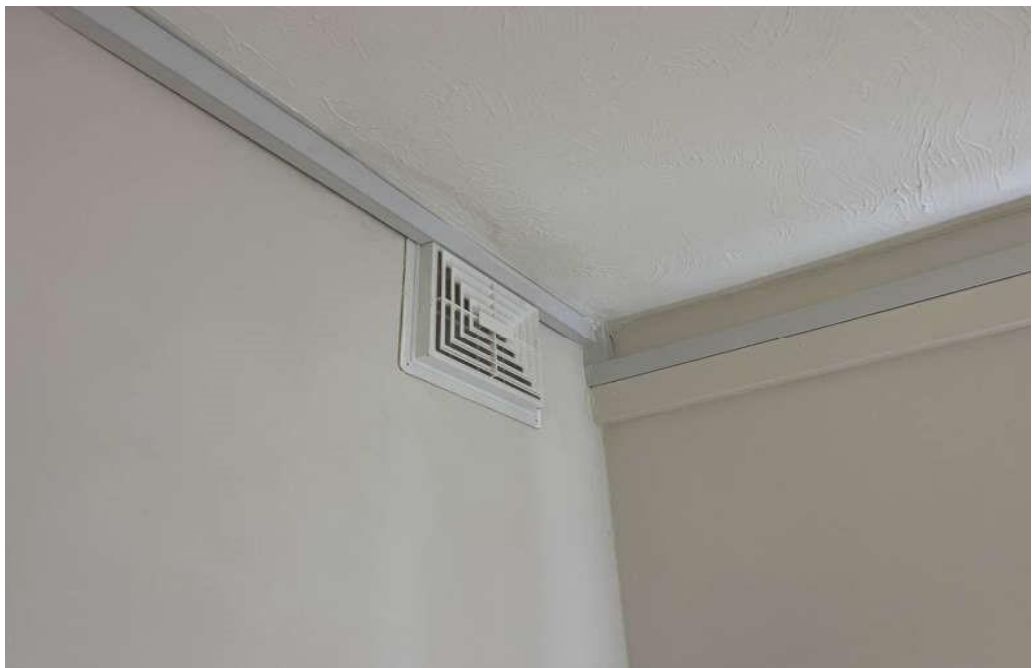
Photograph 13 – Damp staining to North West corner of building at Ground Floor
