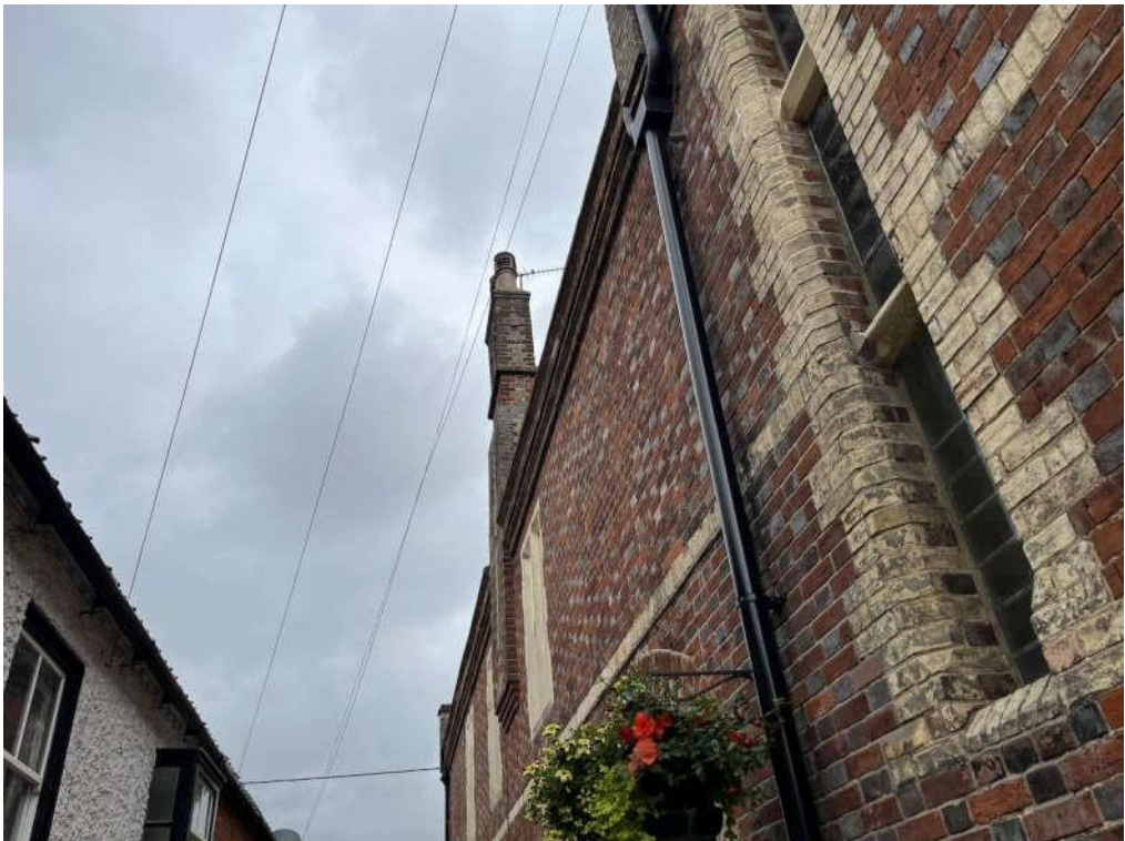
Photograph 11 – ‘Leaning’ chimney looking North.
